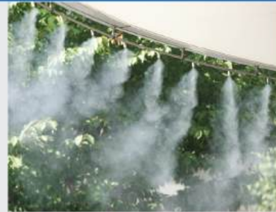
Control dry mist at Mall, Park etc
